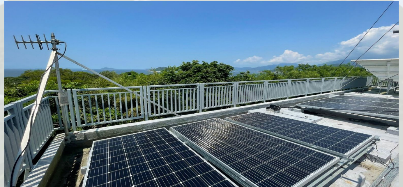
Solar panels in Cheung Chau Meteorological Station
