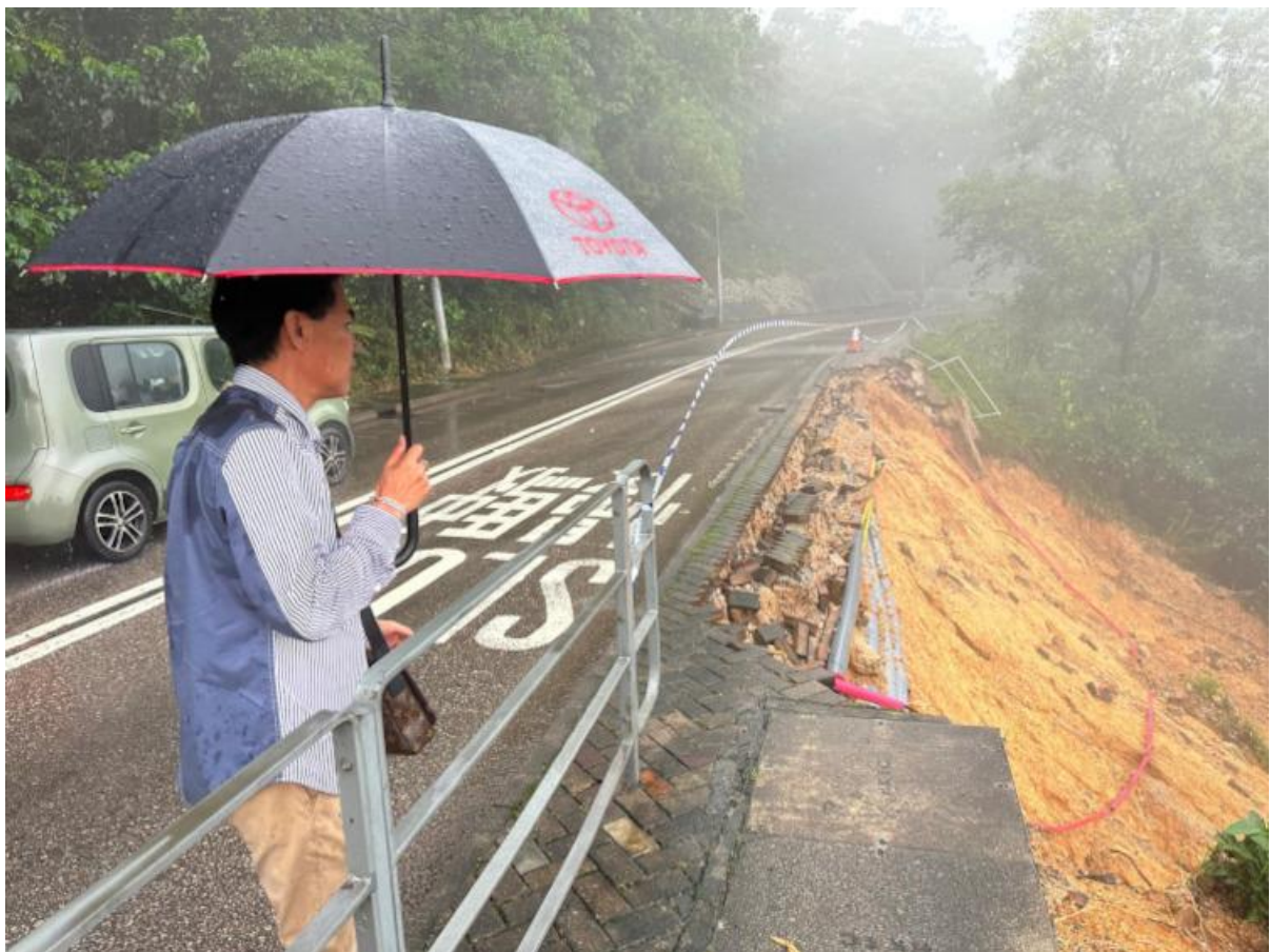
圖 1.4 2024 年 5 月 4 日暴雨期間清水灣道有山泥傾瀉 (鳴謝：坑口鄉事委員會) Figure 1.4 Landslide on Clear Water Bay Road during the rainstorm on 4 May 2024 (Courtesy of Hang Hau Rural Committee)
