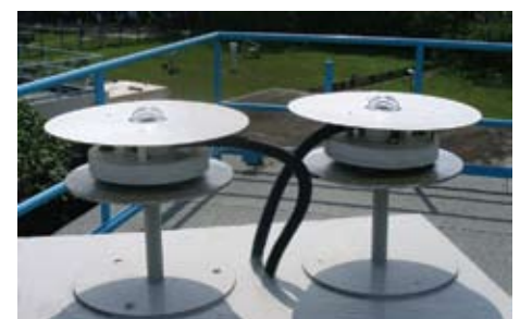
Figure 2: Solar radiation meters installed at King's Park Meteorological Station
