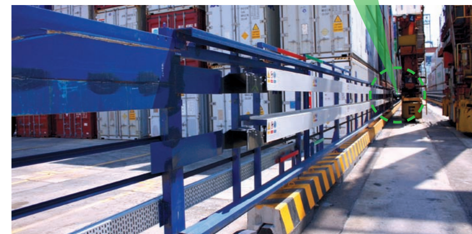
The conductor bar supplying power to the eRTGC and plugging mechanism (inset)
