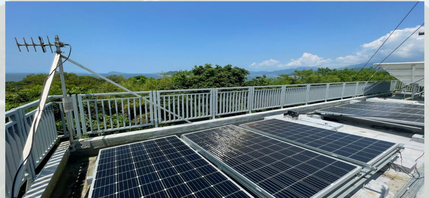
Solar panels in Cheung Chau Meteorological Station
