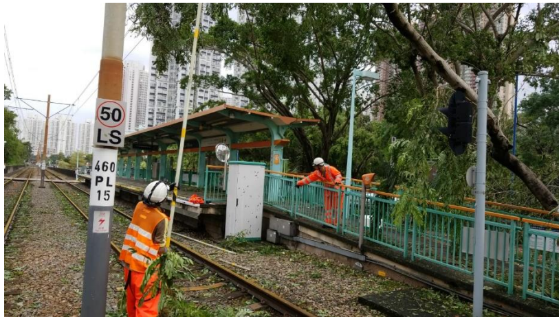
Tree branches entangling the overhead lines
