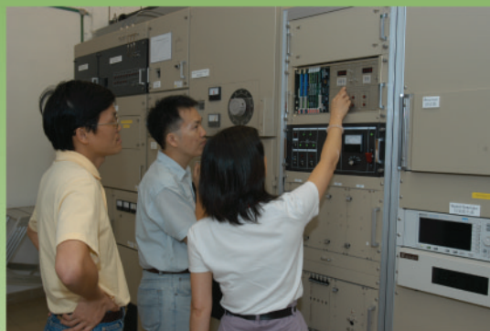
定期檢查天氣雷達的操作 Regular checking of weather radar operation
