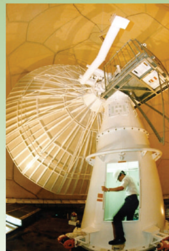
檢查雷達天線確保運作正常 Checking the radar antenna to ensure normal operation
